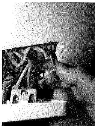
CPC on Lighting circuit has come loose (sorted on
