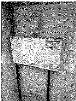
Board tested & compliance stickers installed
