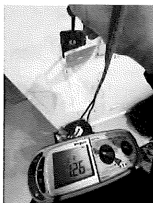
no CPC continuity on lightning circuit C2
