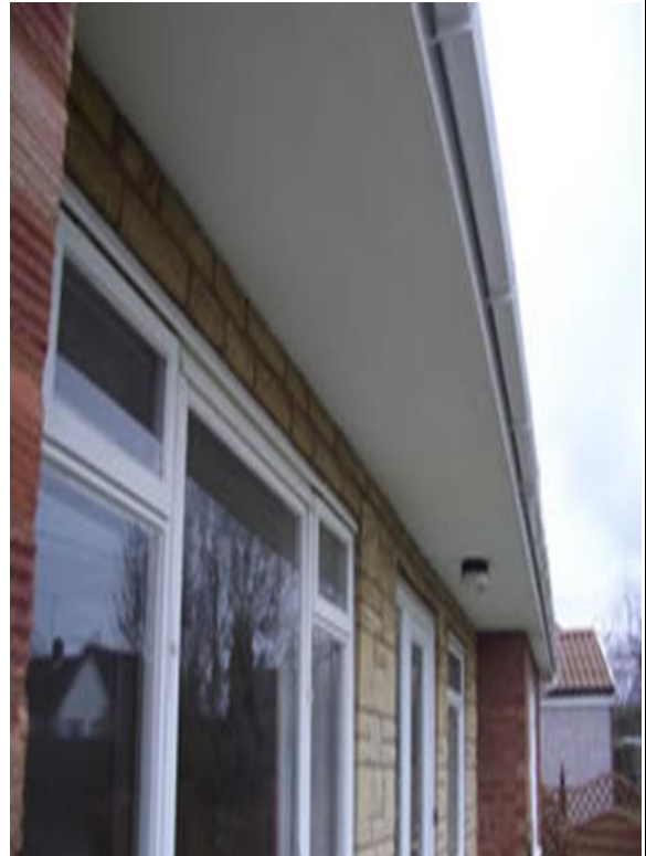
Pieces of Asbestos Insulating Board (AIB)
