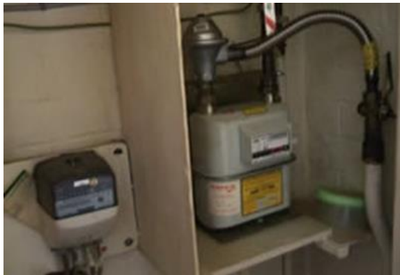
Asbestos panelling around a gas meter
