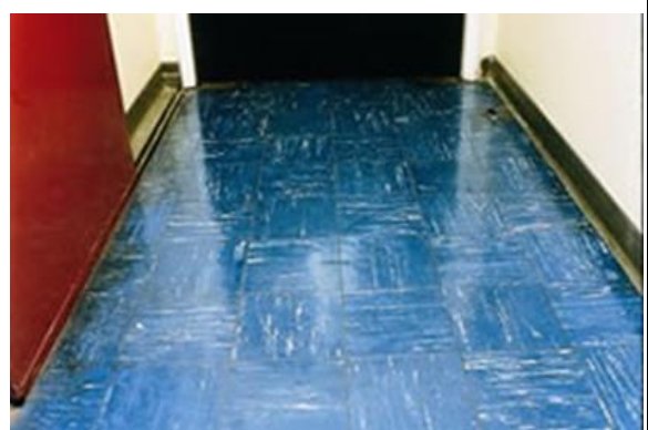
Asbestos containing floor tiles in a corridor
